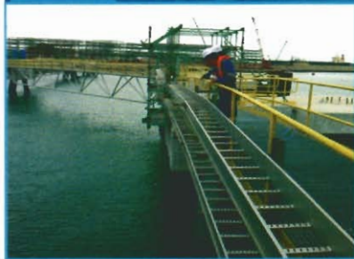
M*RAK cable ladders installed at one of the jetties at SLNG
